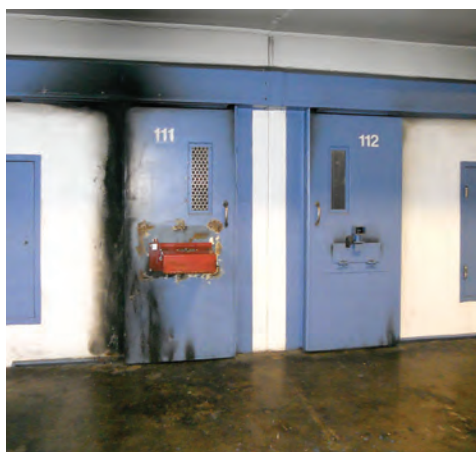
Doors in the solitary confinement zone of EMCF are charred from the fires that otherwise-ignored prisoners routinely set to get the attention of guards in emergencies.
